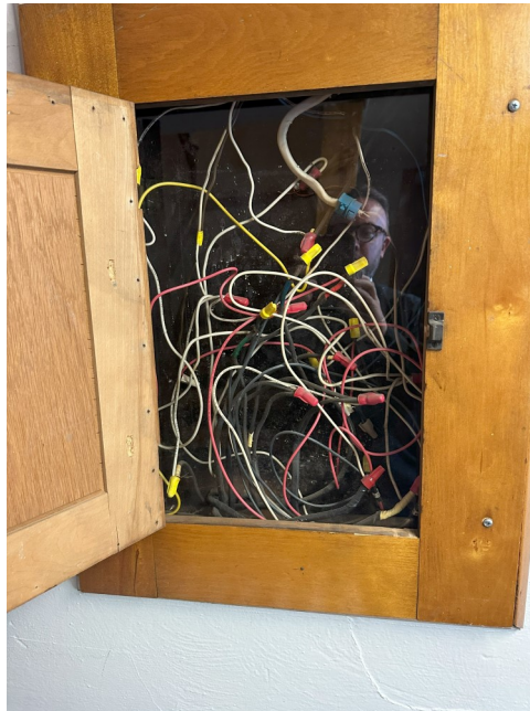
Above: One of SPR's century-old electrical boxes...Looks perfectly safe!
